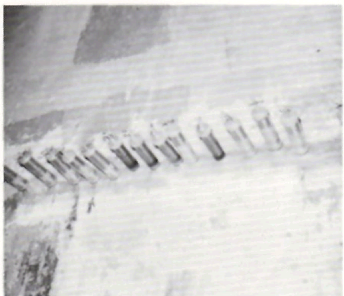
Leaks at an intersection of the perimeter wall pour were epoxy-injected, then recoated and painted.
