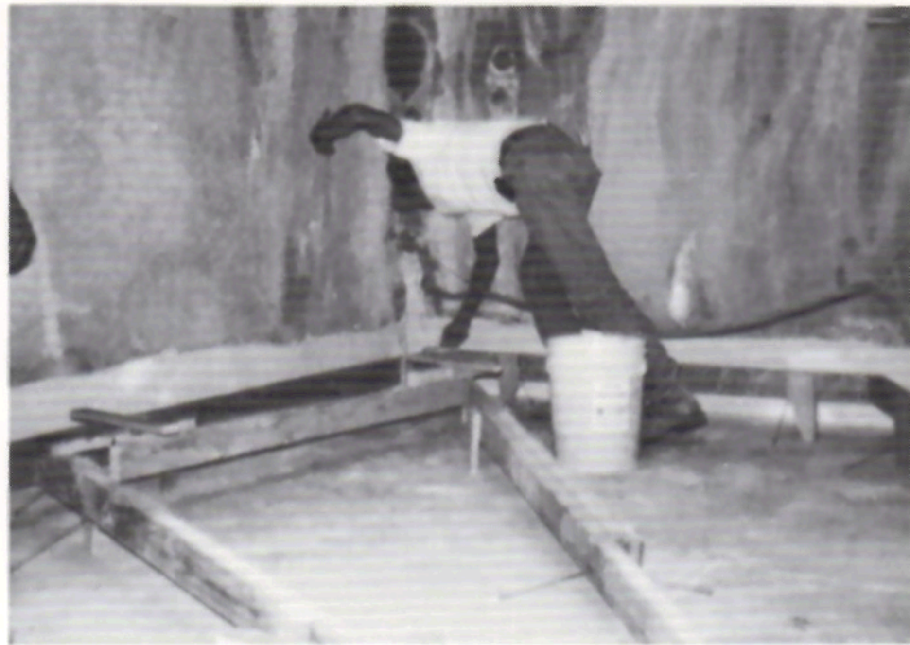
Water-stained vent shafts required patching, injection, recoating and painting. This multi-step process required an elastomeric membrane-coated concrete deck sloped to a new sump pit.
