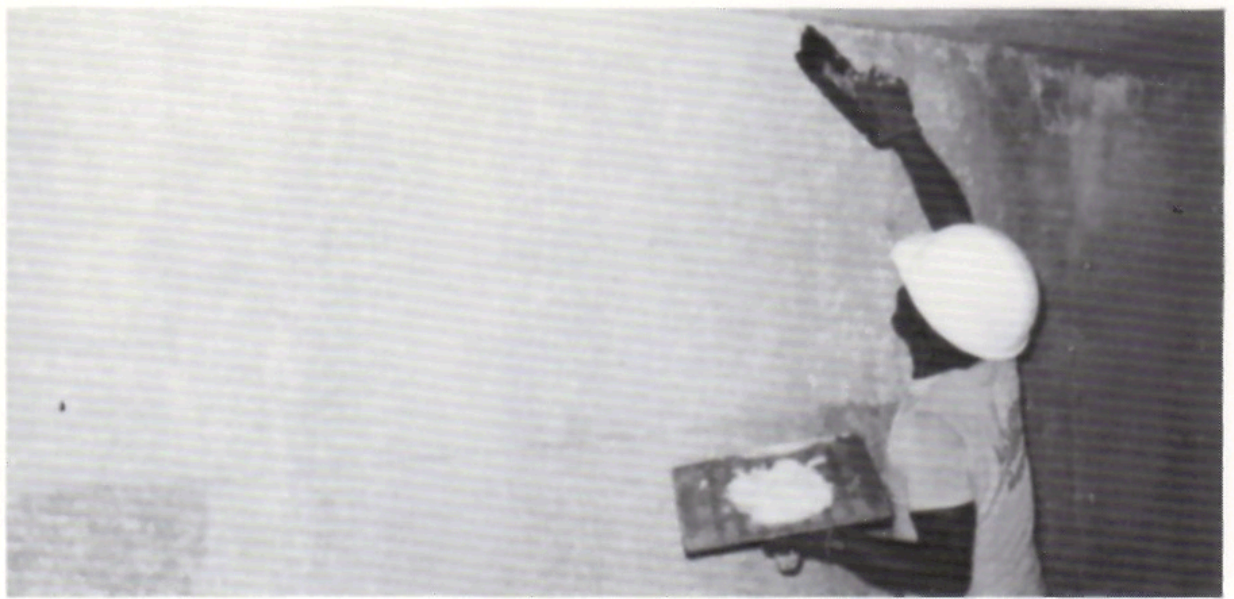
Repairing wall joints required a multi-step process of chipping away damaged concrete, using a cementitious hydraulic filler as a water plug, applying several different types of epoxy mortars and coatings, then repainting the area.
