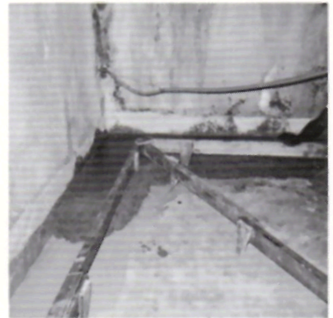
A detail of the vent shaft area, showing new concrete forms in place.
